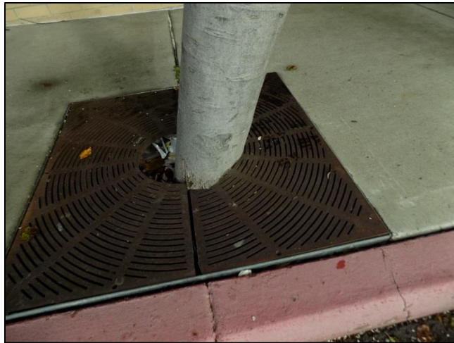
Photo 5 – Southern magnolia #5 (as well as several others) was being girdled by the grate covering the tree well.
